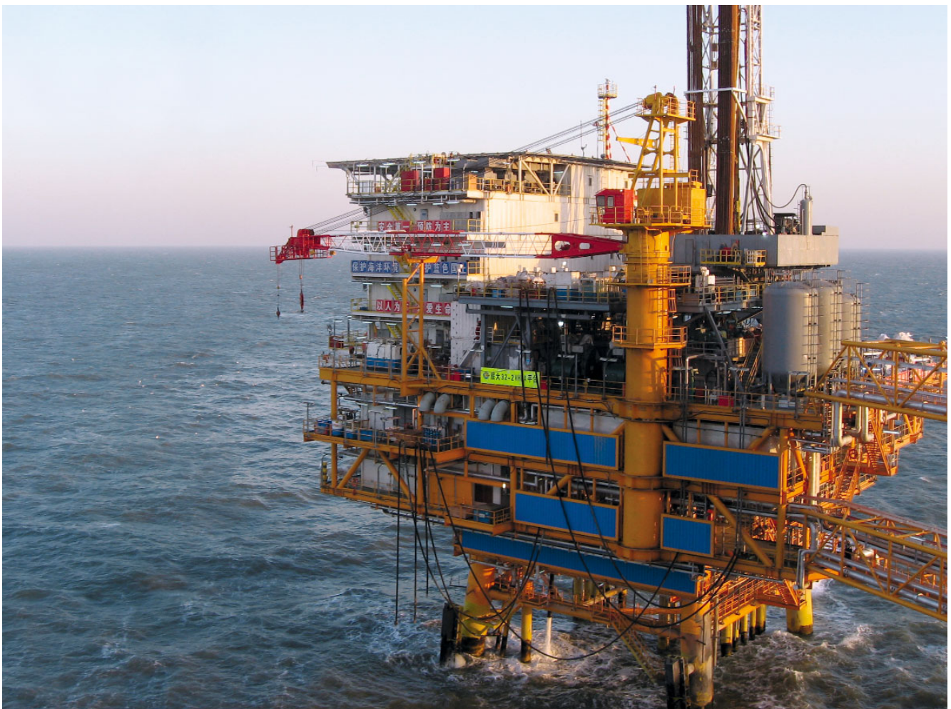
Two RGMS70/2 burners with digital combustion management provide the necessary process heat on the oil production platform CNOOC LUDA 27-2
