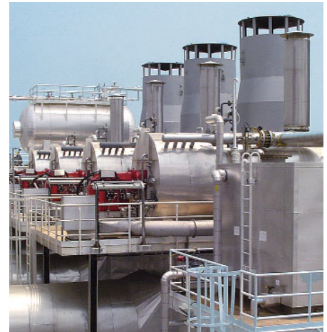
Four RGL70 burners on thermal fluid heaters ensure that the crude oil can be pumped
